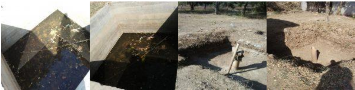
Pit for Disposal of Waste Water
